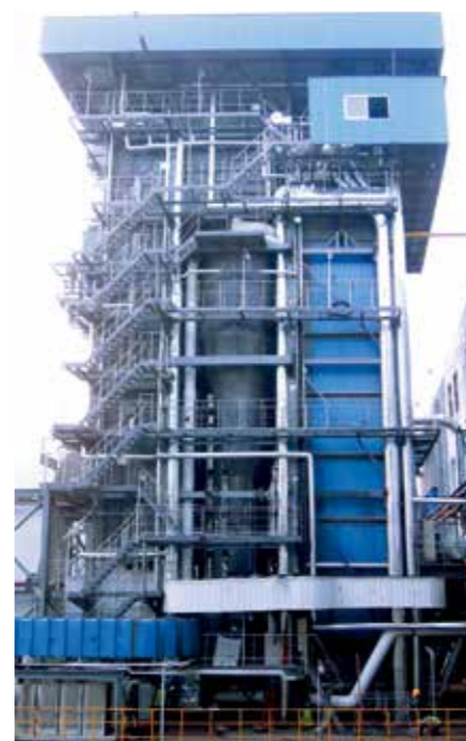
山东兖州 75 吨 / 时高温后燃循环流化床锅炉 75 t/h CFB Boiler with High Temperature and Post-Combustion in Shandong Province
