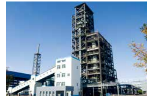
甘肃金化千吨级加压循环流化床气化炉 Pressurized CFB Gasifier with the Capacity of Kiloton/day Grade in Gansu Province
